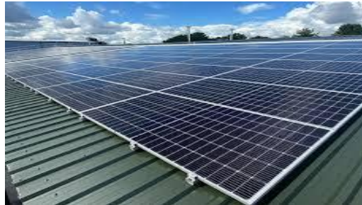
Fig:7 PV solar panel
